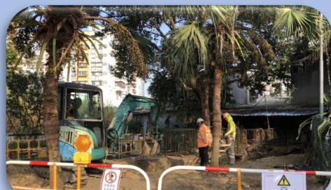
於菜園角村敷設污水渠道 (進行中) Sewerage Works at Tsoi Yuen Kok Village (In Progress)
