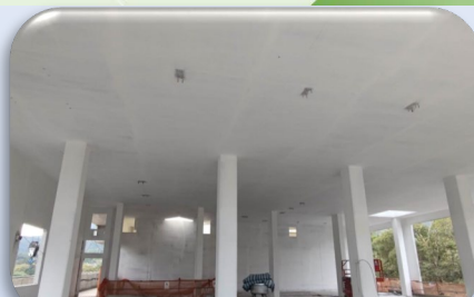
新沙頭角污水處理廠 (完成結構工程) New Sha Tau Kok Sewage Treatment Works (Completion of Structural Works)
